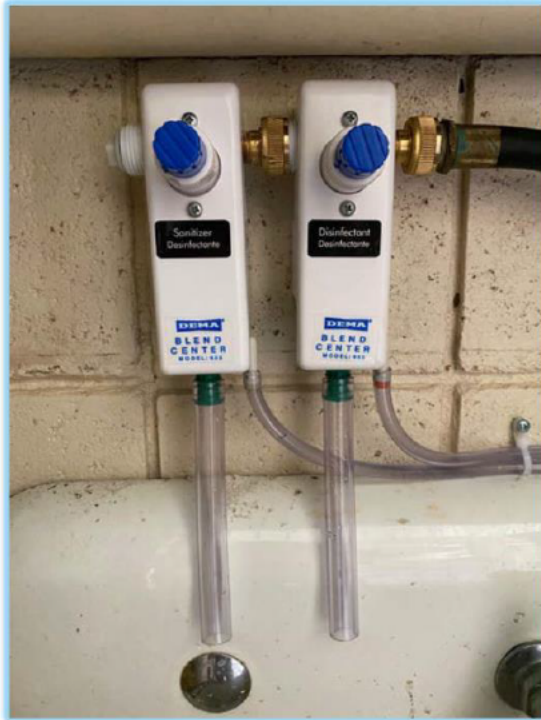
Figure 1. Sanitizer and Disinfectant proportioners installed for proper dilution of cleaner.
